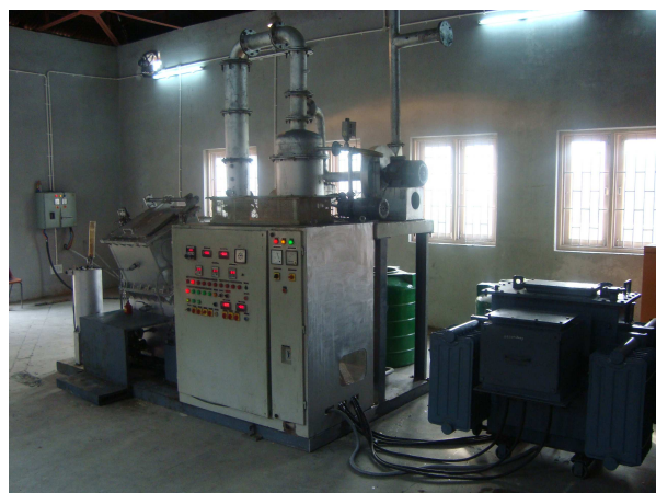
Photograph of Plasma Pyrolysis system installed in Srinagar
